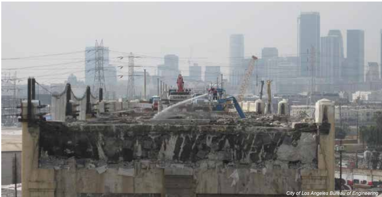
Sixth Street Viaduct Demolition as of March 16, 2016. The $449 million project to replace the beloved bridge, the Sixth Street Viaduct Replacement Project, is the largest bridge project in the history of Los Angeles. With funding from the Federal Highway Transportation Administration and CALTrans, the project is being led by the City's award-winning Bureau of Engineering.
