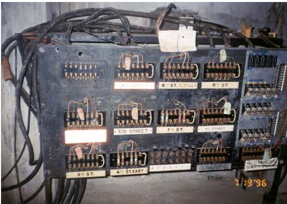
Signal system control in Pershing Square room, 1952 Graphic - 3092
